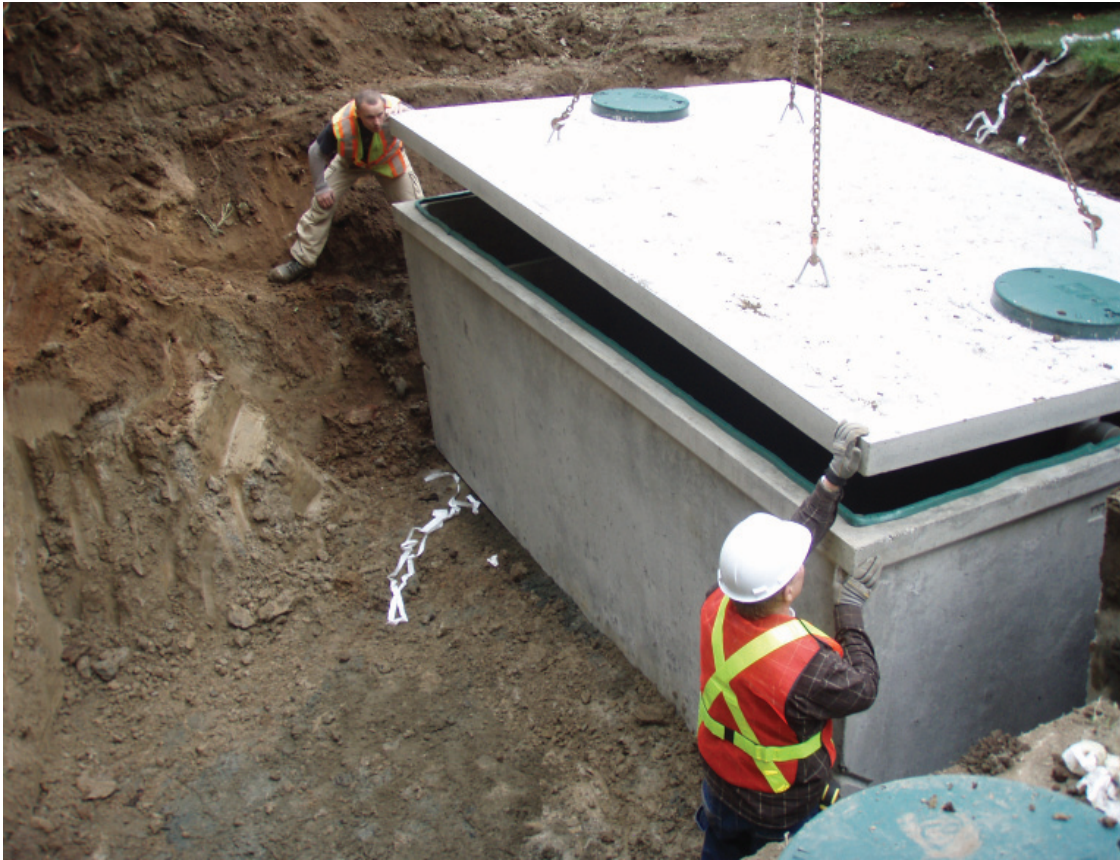
WOWTC Students Installing Septic Tank Lid Reprinted with permission of John Hayton
