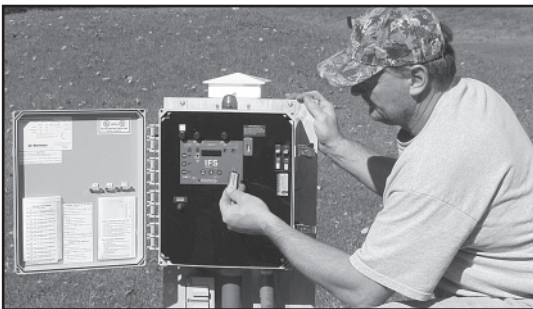
IFS In-Site™ Event Monitoring Control Panel
